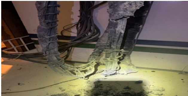
Figure 1 - Fire Damage to Compressed Air Hoses and Heat Tracing Cable
